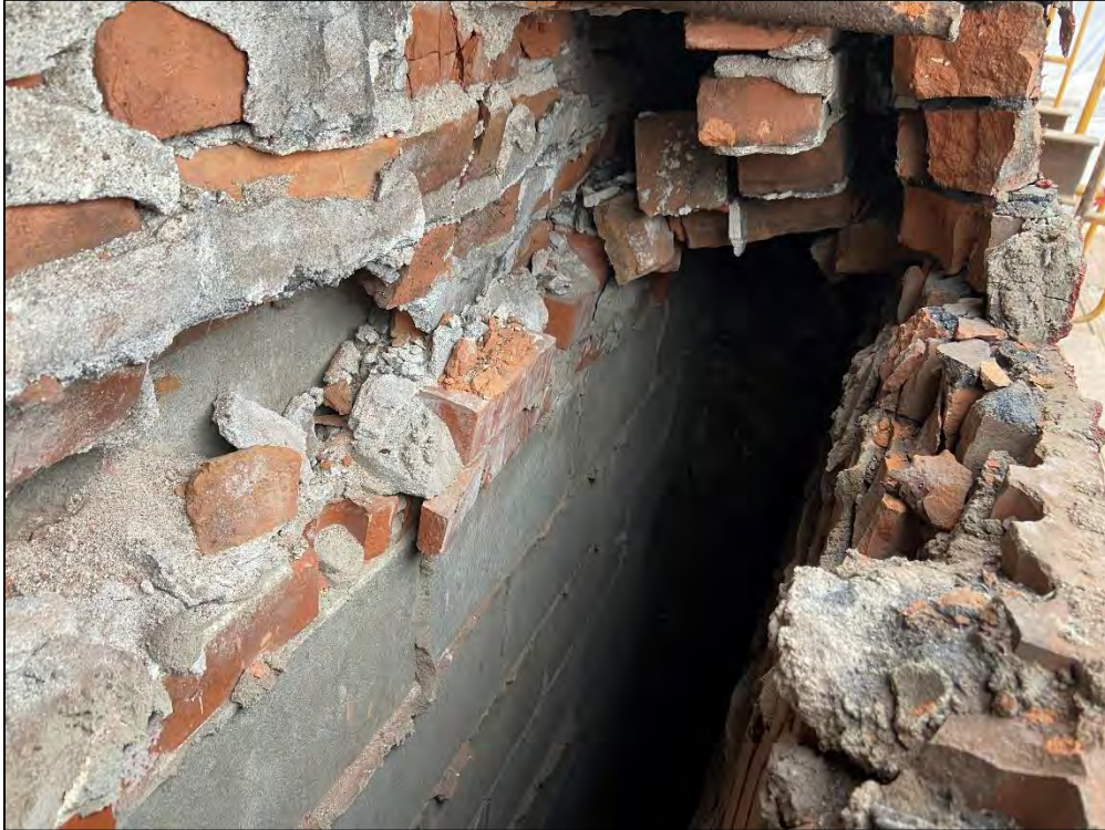
Photo 1 – Void between CMU and Clay Brick Façade
