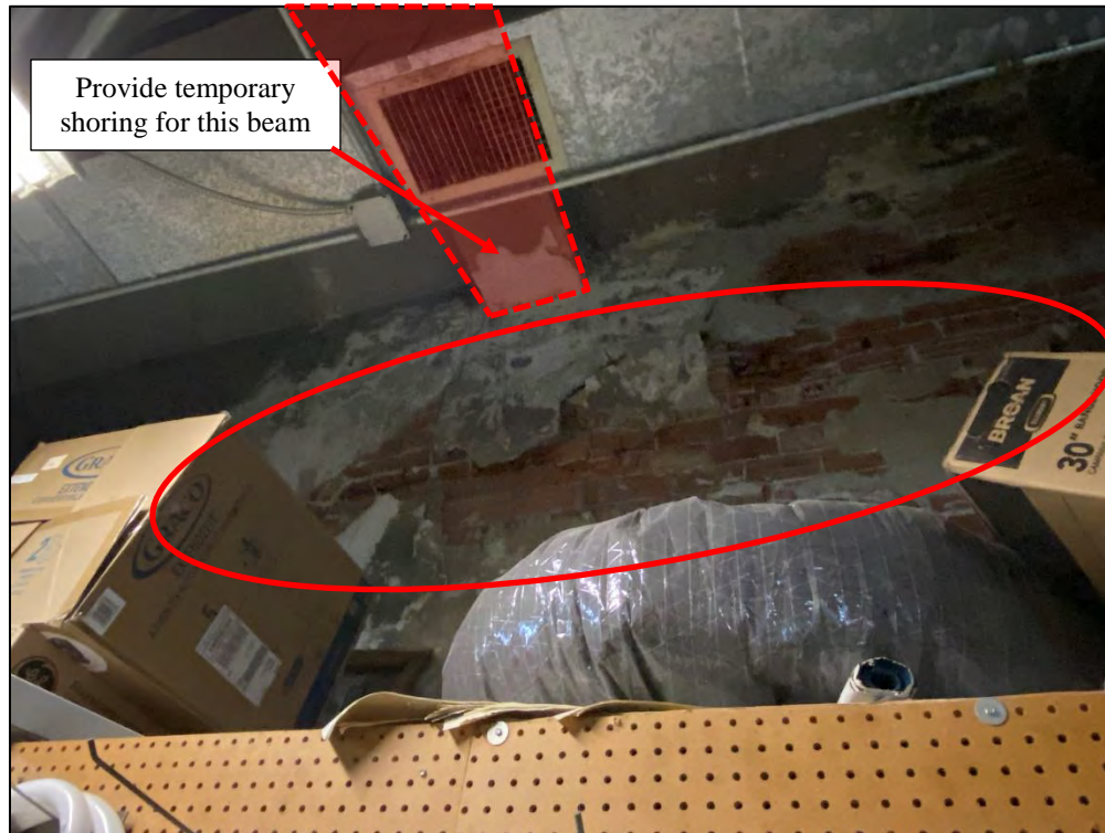
Photo 1 – Damaged Brick & Beam to Support
